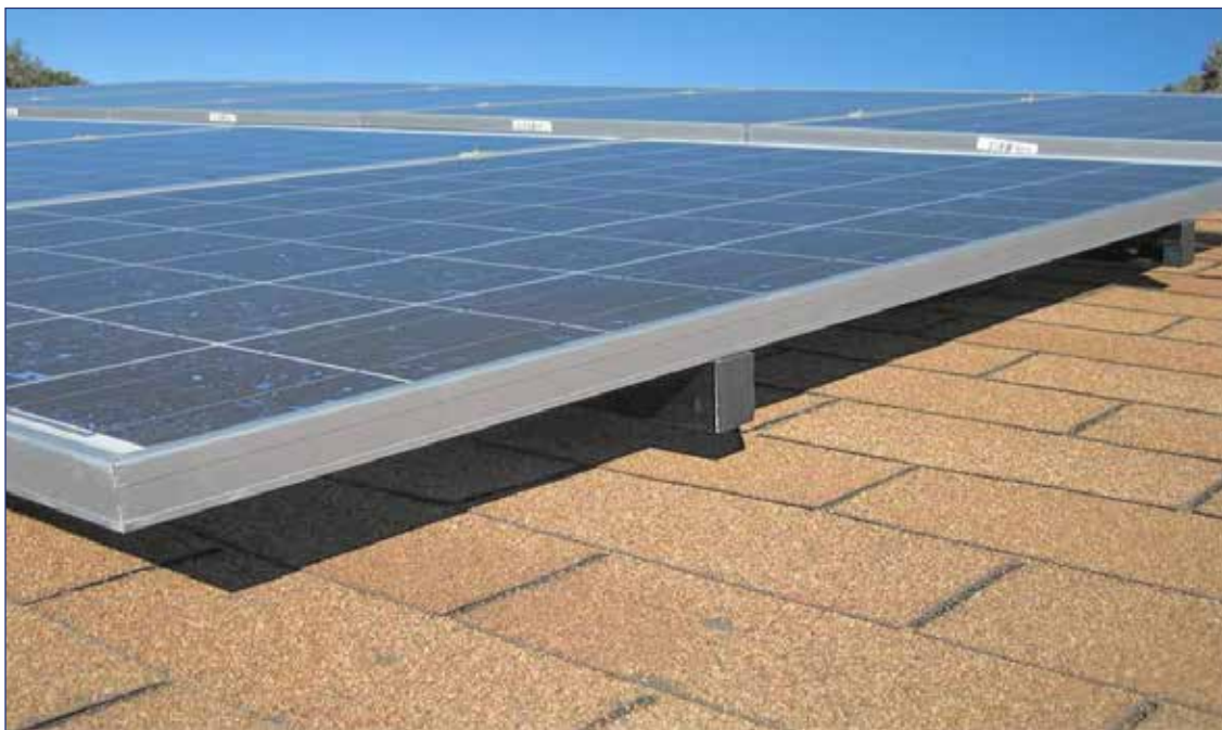
Edge of array with end caps in rails
