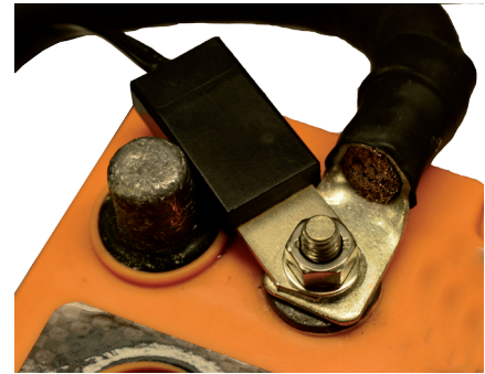
Fig 2.5(b) Temperature Sensor Installation
