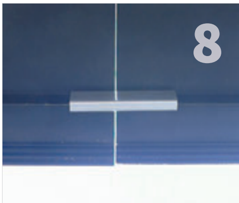
Install remaining skirt sections. Use skirt clips as needed to maintain alignment at skirt junctions.
