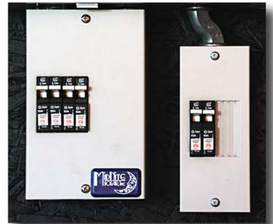
Photograph showing the Big Baby Enclosure and the Baby Box installed.
