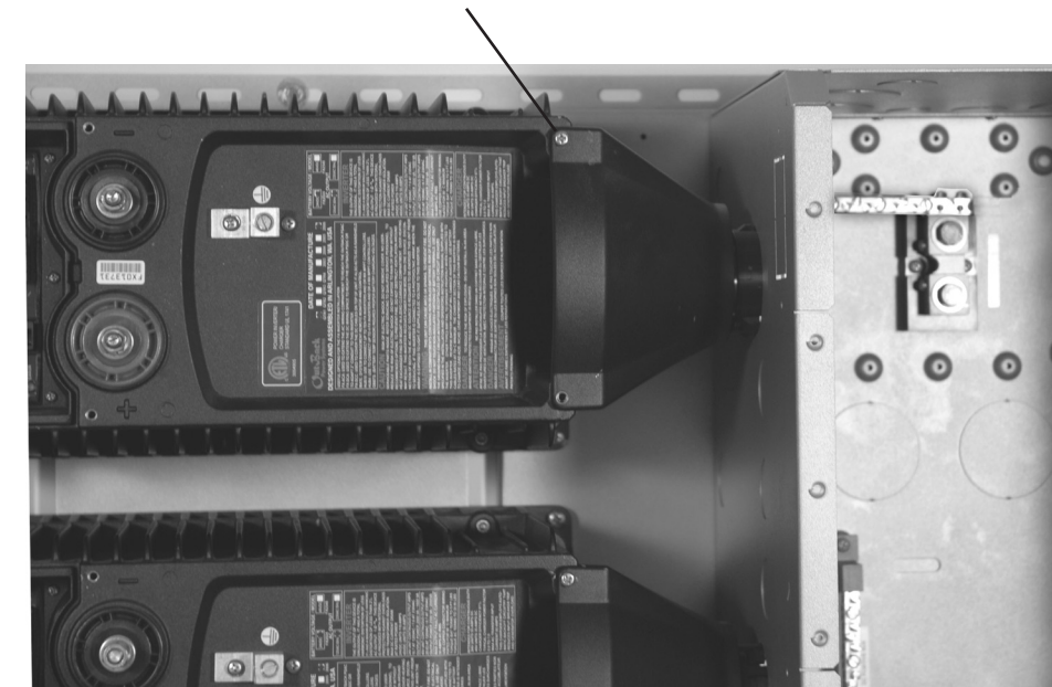
Figure 10: DCA in place
