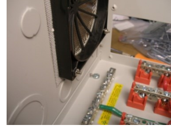
E-Panel earth ground bus (AC & DC)
