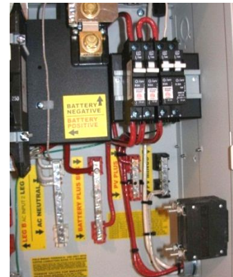
63 amp din rail DC-GFP wired with a 63 amp PV disconnect and a 63 amp controller output breaker.
