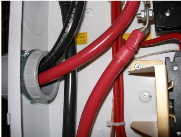
Wire exit to inverter
