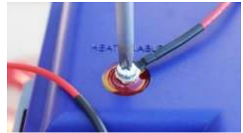
Figure 13: #8 ring terminal onto the heater enable post
